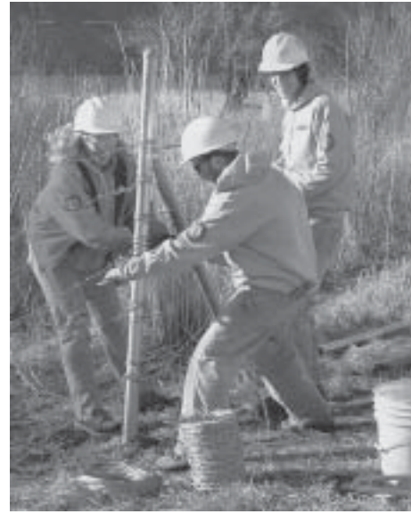
Building riparian fencing at Lmumma Creek. L-R: Rhyan Grech, Doug Jewell, Tom Orvis.
